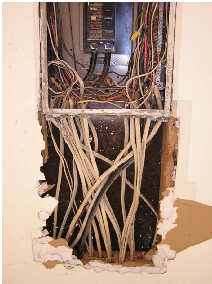
Fig. 6 – NM Cables From House VA-3
