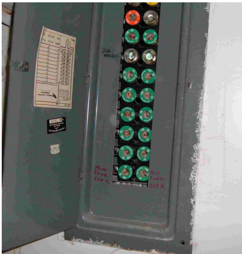
Fig. 12 – 30 Amp Fuses From House AL-8
