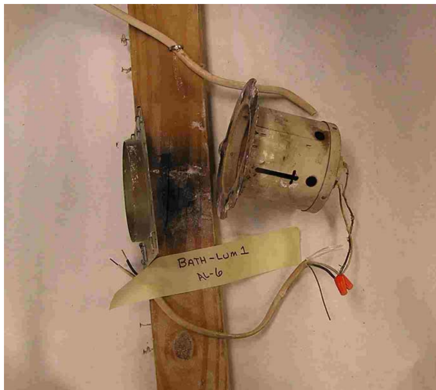
Fig. 22 – Recessed Luminaire From House AL-6
