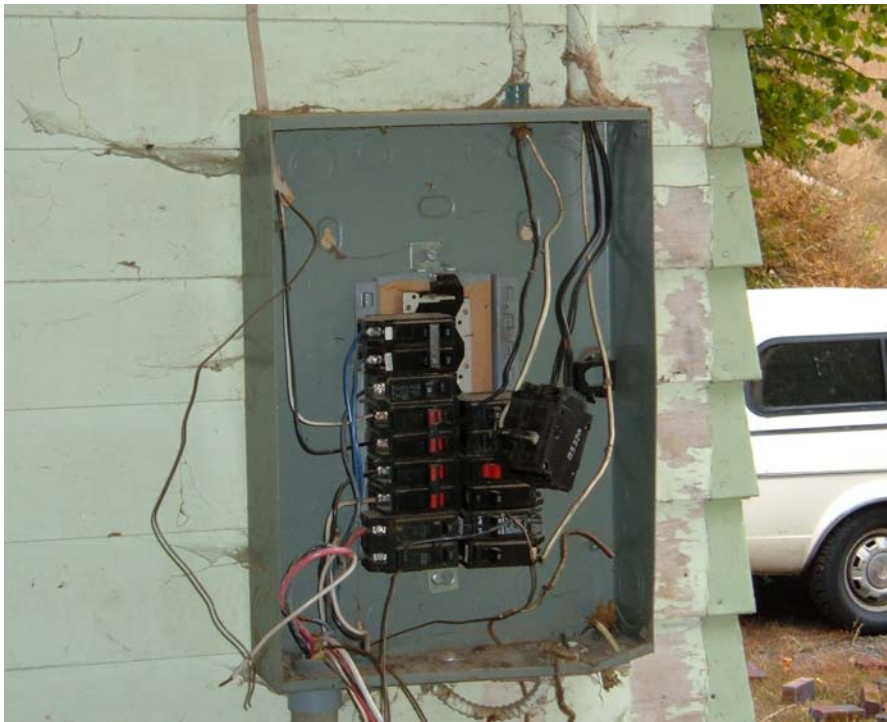
Fig. 30 – House OR-1, Main Disconnect Outdoors
