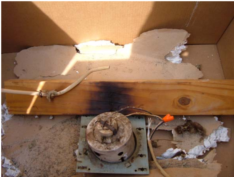
Fig. 43b – House AL-6, Recovered Recessed Ceiling Luminaire
