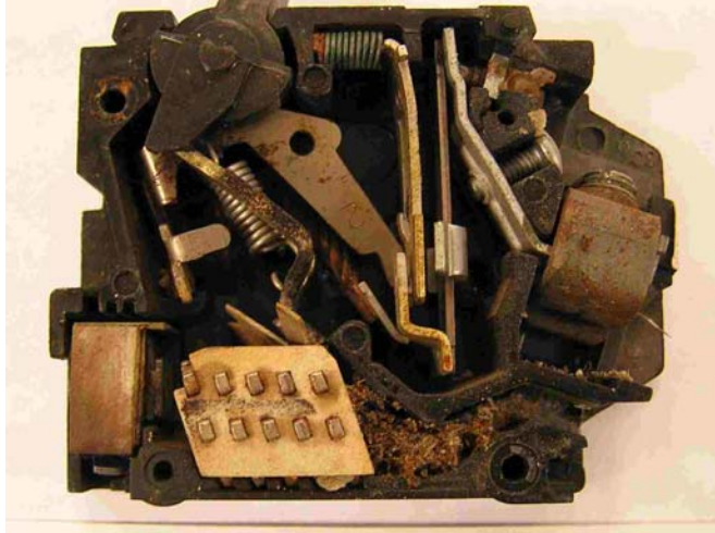
Fig. 15 –House AL-8 Breaker 9-11, Corrosion Damage
