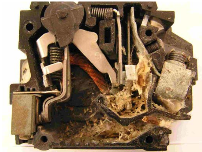
Fig. 16 –House AL-9 Breaker 5-7, Insect Nesting
