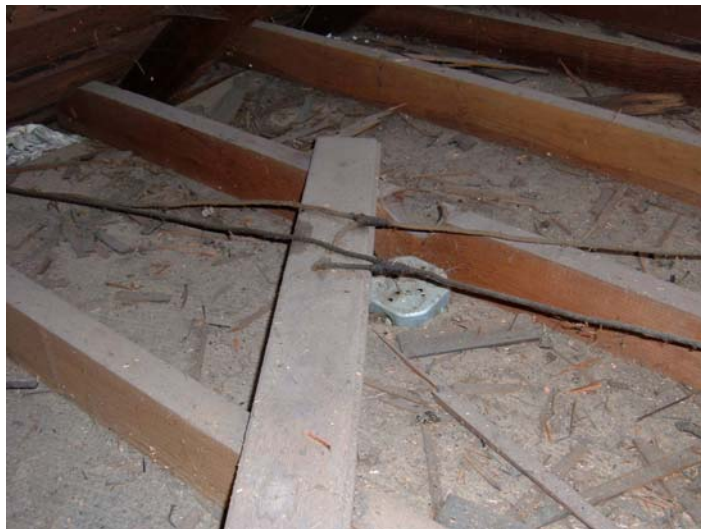
Fig. 2 – Knob-and-Tube Wiring From House OR-1
