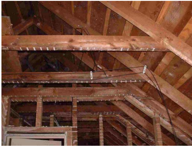
Fig. 1b – Knob-and-Tube Wiring From House IL-6
