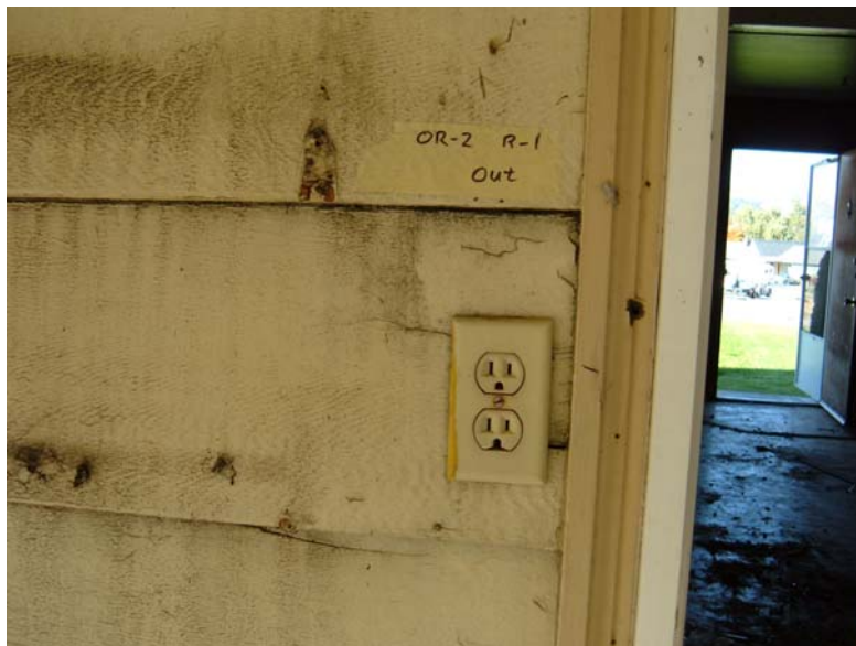
Fig. 42 – House OR-2, Open Receptacle Outdoors
