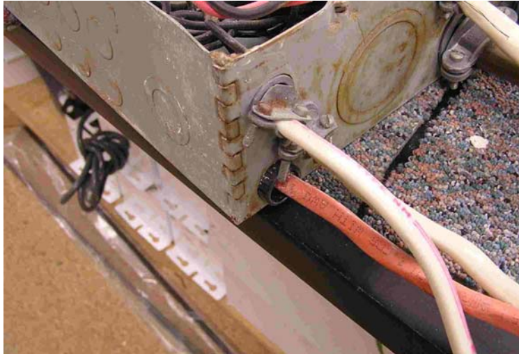
Fig. 36 – House MA-3, Cable Clamp Not Provided
