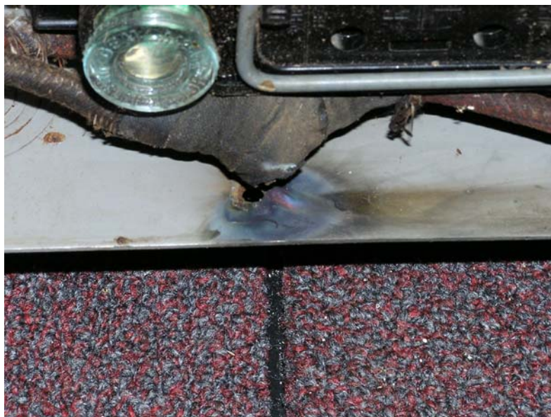
Fig. 9 – Arcing at Conductor Splice at House WI-1
