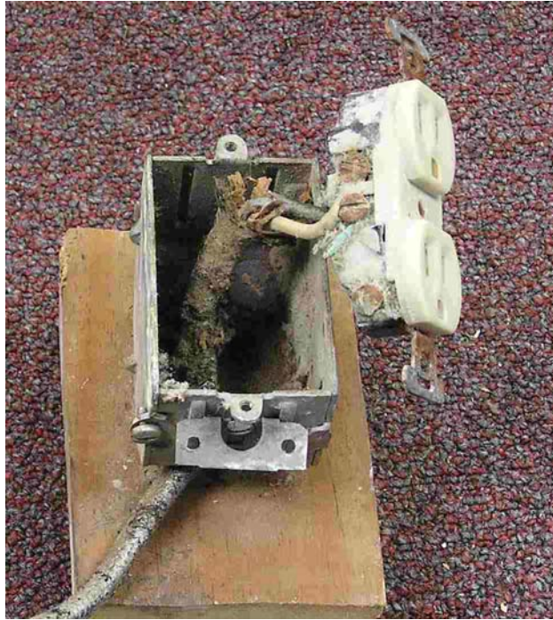
Fig. 41 – House AL-4, Grounding Type Receptacle Without Ground
