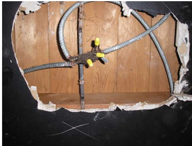
Fig. 35 – House WI-1, Open Splices in Ceiling
