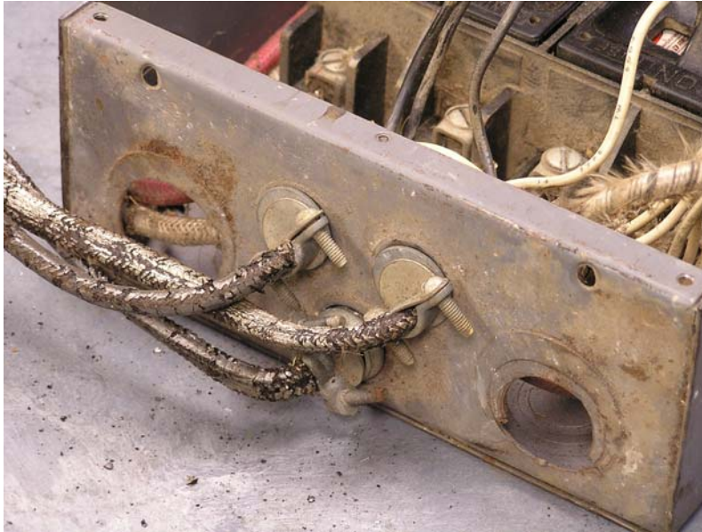
Fig. 27 – House AL-3, Unused Openings in Enclosure
