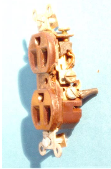
Figure 1 - A Receptacle Damaged by a Glowing Connection
